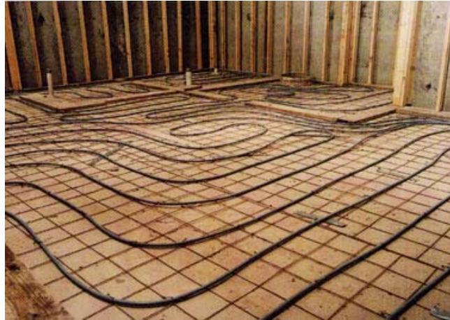
Figure 2-G. A Radiant floor system provided an attractive solution for the project.
